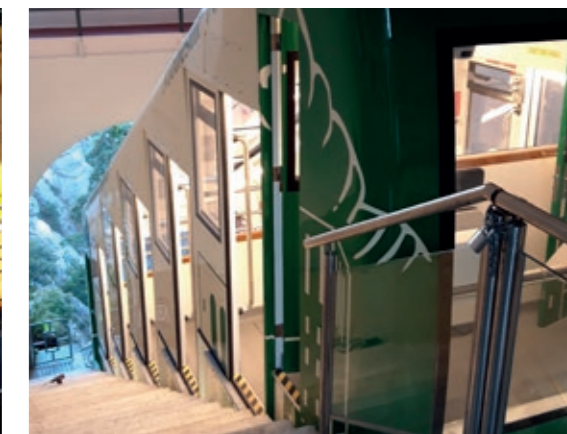
LEITNER SpA – Telefericos Y Nieve - Compocel AL Cable car -work in progress
