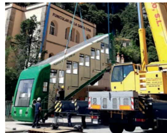
LEITNER SpA – Telefericos Y Nieve - Compocel AL Wagon at cable car lift departure
